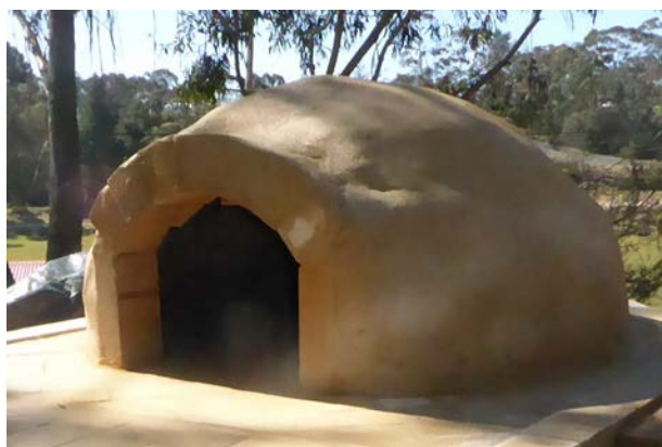
The woodfired oven is starting to look the part, but will soon sprout a chimney stack.
